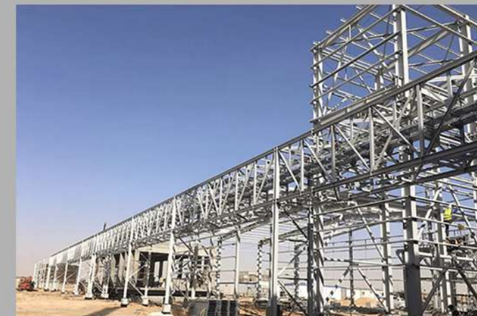
OIL & GAS SERVICES (ONSHORE PLANTS, OFFSHORE PLATFORMS)
